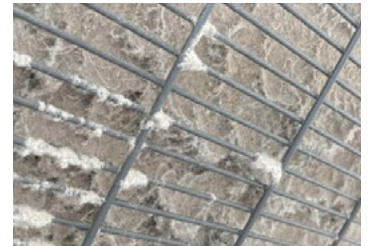
Severely Neglected Condenser Coil
