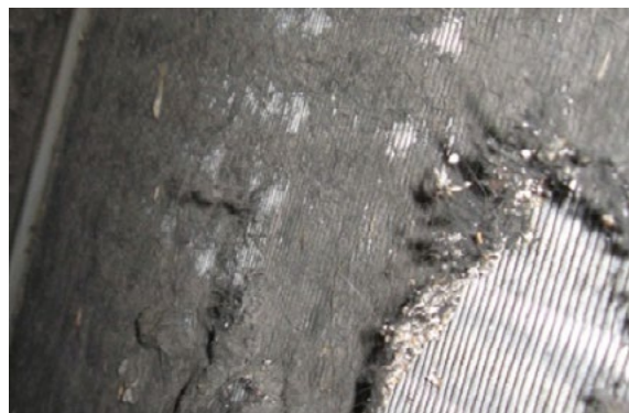
2 years without maintenance
