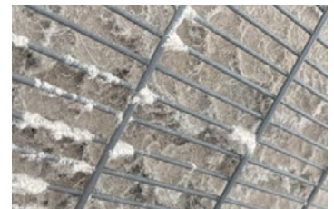
Severely Neglected Condenser Coil
